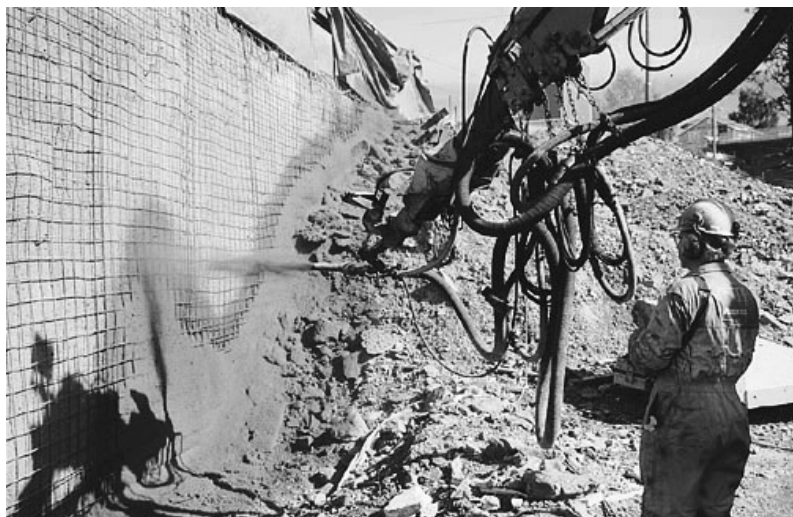
Figure 4 Sprayed concrete with recycled aggregates (0-4 mm) at the Gaustabekk Building site (Picture: Bente Lillestøl, Veidekke ASA)
